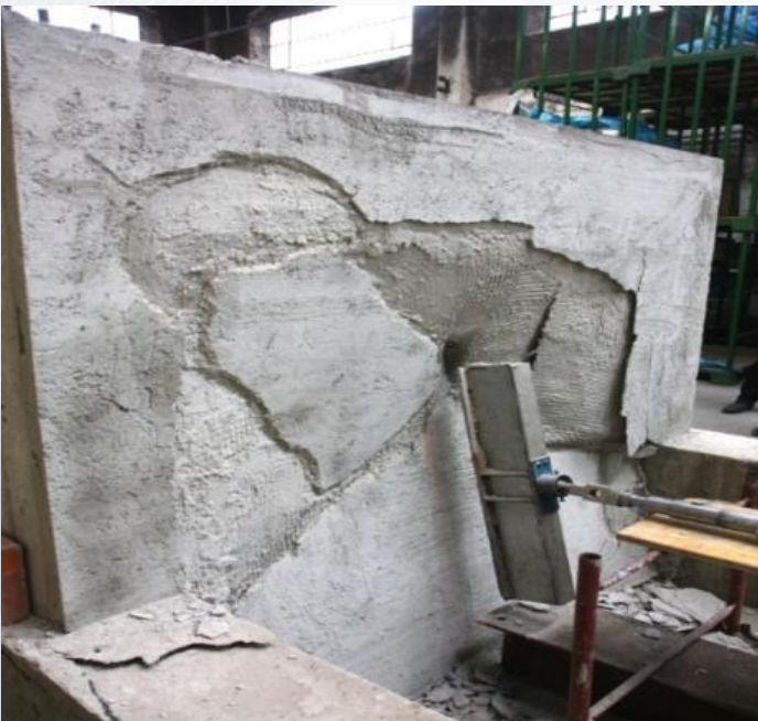
Partition wall with force on the side with Aegis in cement plaster.
