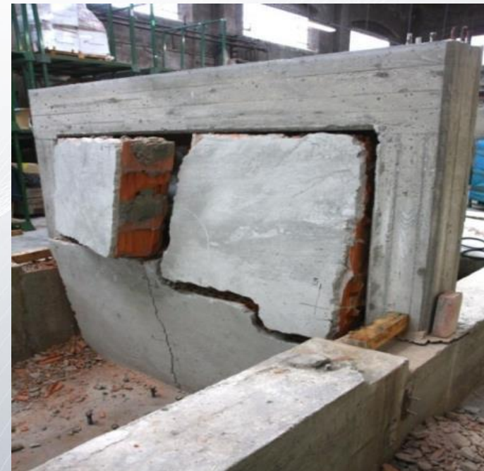
Side opposite to Aegis, no contact with columns or beams. Breakage but no falling of wall parts
